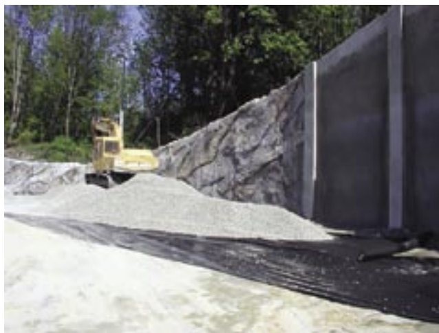
Fig. 5: Snohomish County Waste Transfer Station, Mountlake Terrace, WA. This wall was originally specified as cast in place
